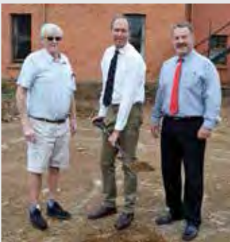
Construction of the 'new' Shepstone House has begun. Mr Craig MacKenzie, Chairman of the Governing Body, was on site with Mr Ken Hackland (left) and Mr Chris Luman (right) to symbolically turn the earth and thereby 'open' the site.
